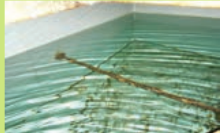
Light debris but corrosion to restraining bars
