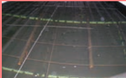
Heavy debris and corrosion of internal parts that will require remedial works
